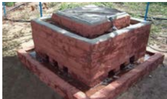
FIGURE 52 Evidence of the use of above-ground Zero Energy Cool Chambers (ZECCs) in the hot-dry climatic zone of India 97
