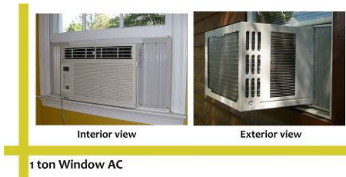
Figure 27. Window air conditioner
