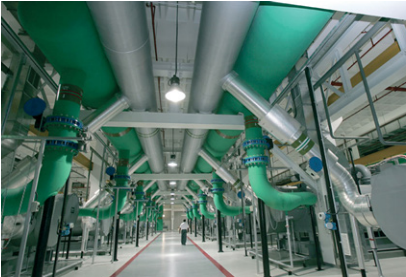
Figure 50b: Water Chilling Plant for a District Cooling System
