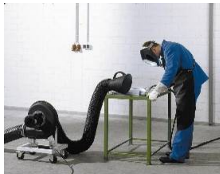
Figure 15: Mobile LEV with flexible duct
