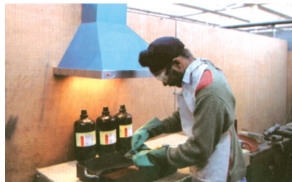
Picture 12: Local Exhaust Ventilation
